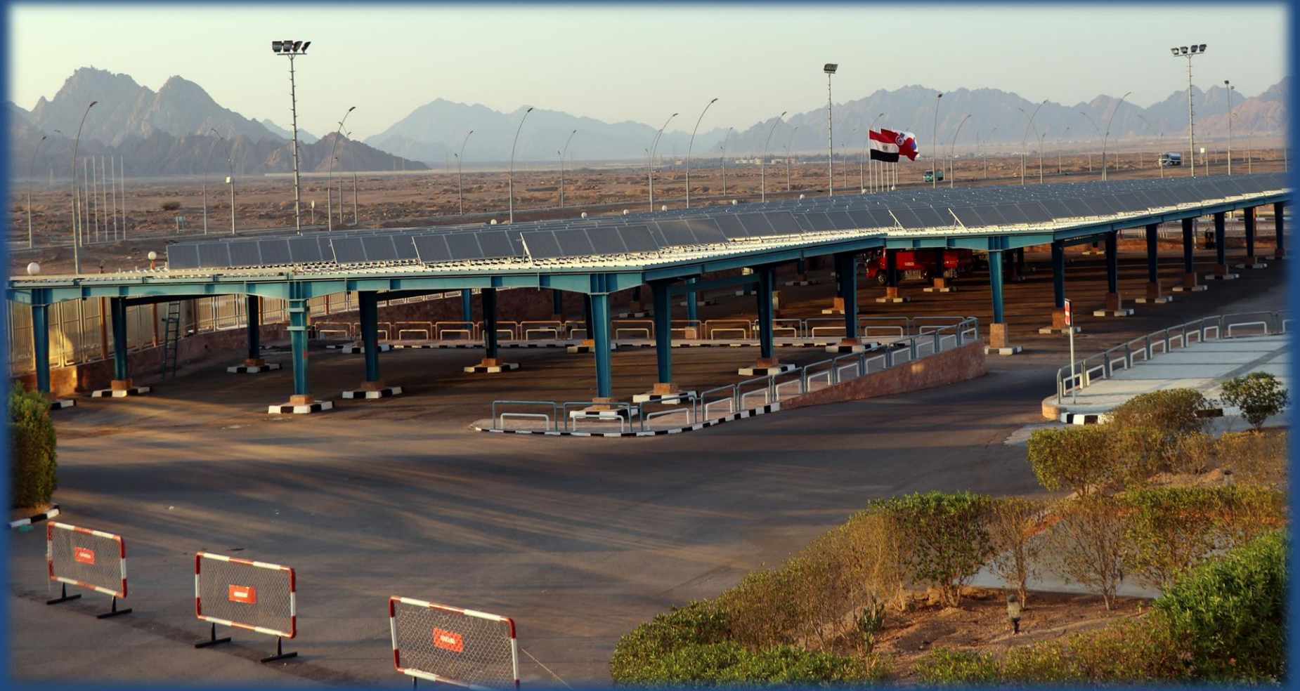
Solar Energy Plant – Sharm El Sheikh
